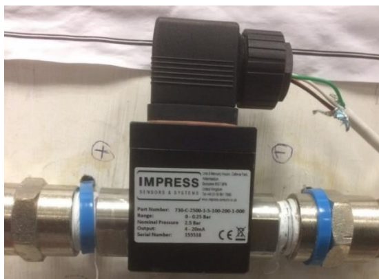
Figure 3.3. Differential pressure transmitter.
