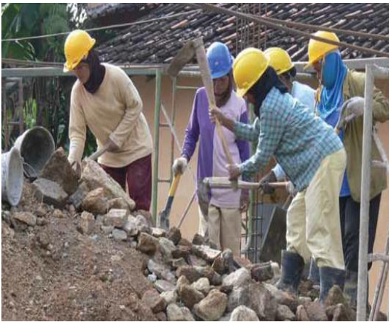
Women work in house reconstruction: they are not only paid but also learn how to build safe and secure house
