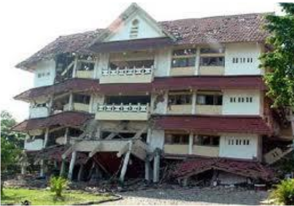
Government office damage from Bantul earthquake
