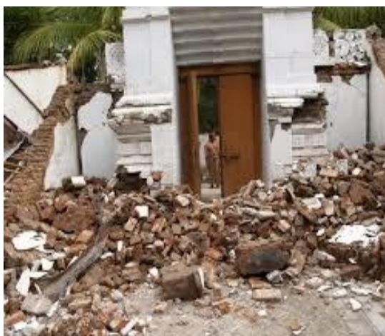
Houses damages from Sleman earthquake
