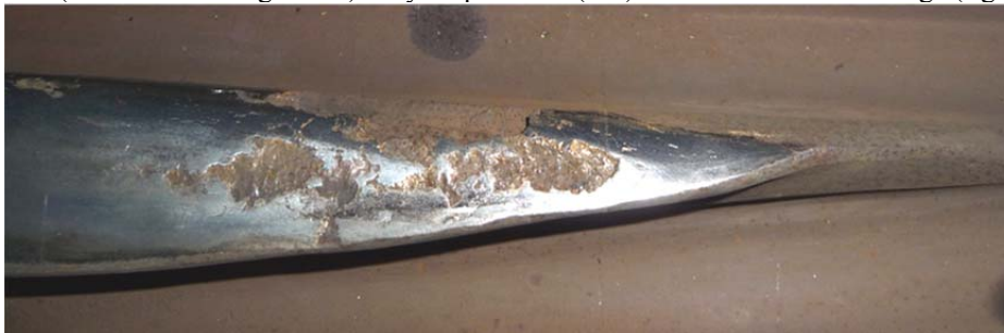
Figure 14. crossing nose showing heavy plastic deformation and distorted nose under the impact of passing wheels (non-compliance of wheel-crossing geometry)
