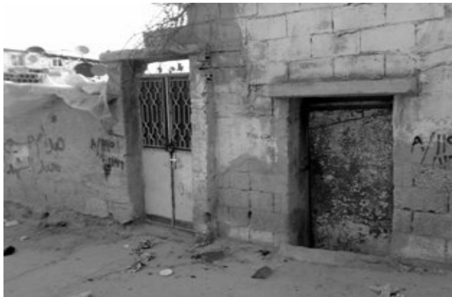
Figure 1 Poor External Appearance
