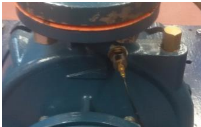
Figure 6-13 Vibration transducer mounted on the pump
