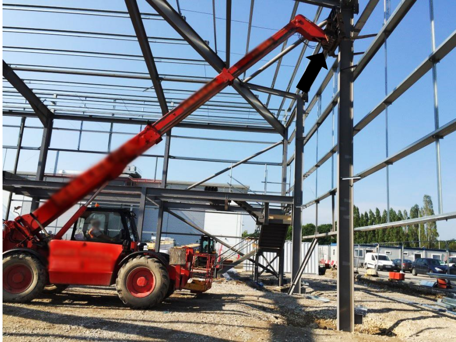
Figure 4-48. A forklift truck was used to pull the second erected side of the building towards north
