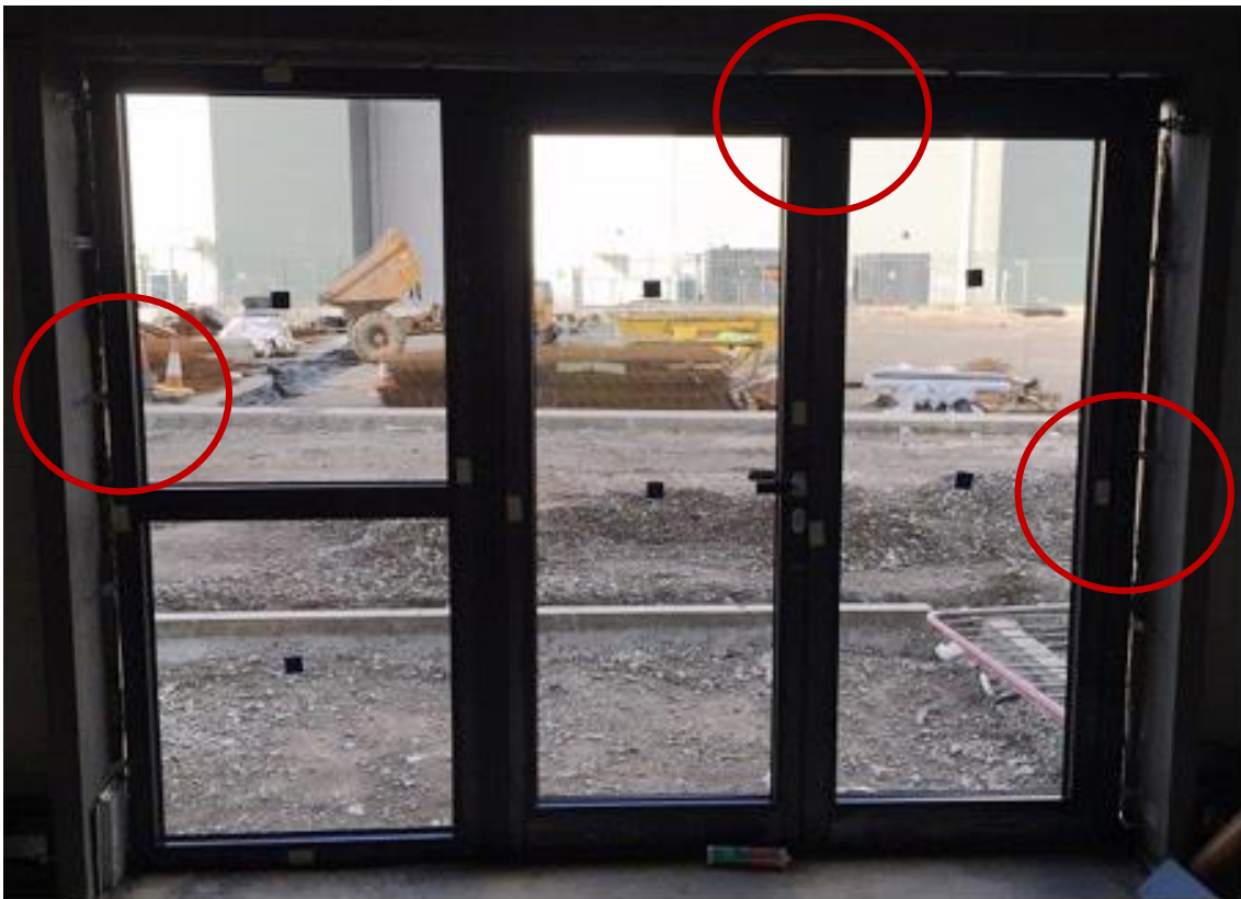
Figure 4-53. The personnel door and gaps around the doorframe
