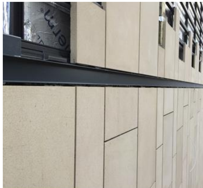
Figure 4-23. Elevation 9 and sagging stone panels
