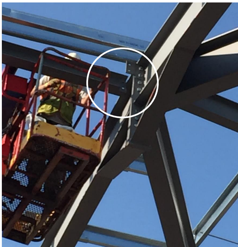
Figure 4-47. The beam between the Gridlines 28E and 30E had an overlap in Gridline 30E
