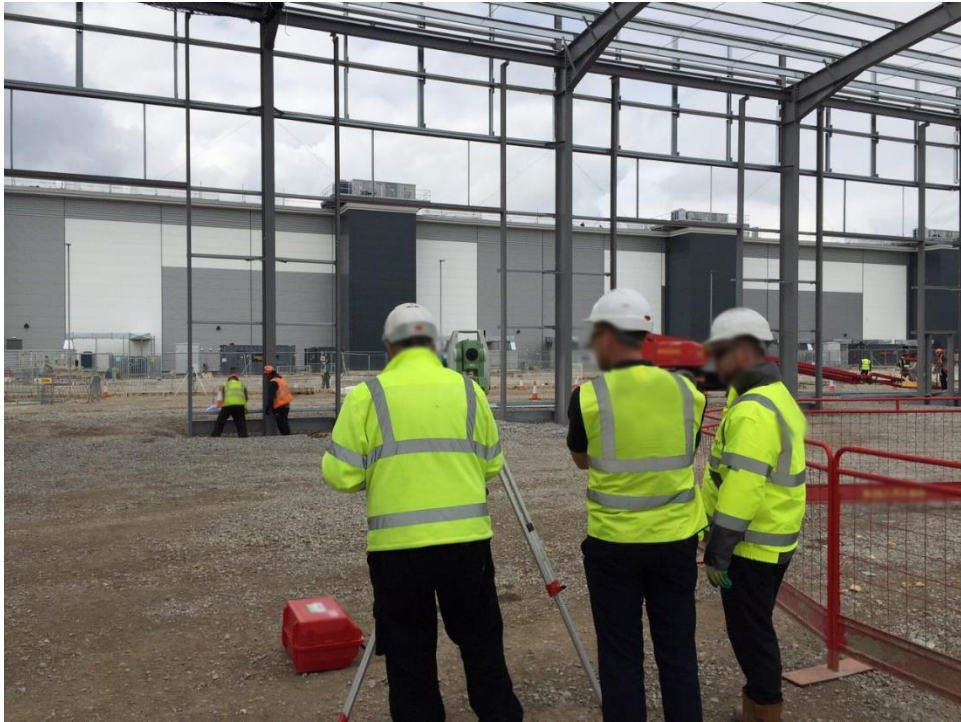
Figure 4-28. The interaction between the site engineer and the steel erector to plumb and level the columns
