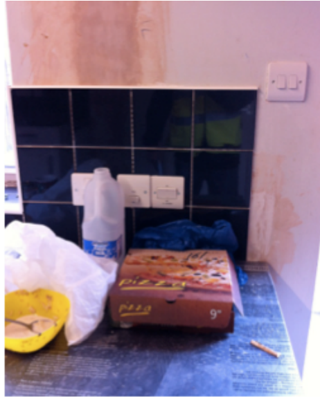
Figure 21 – Light switch (top right) fitted in a wrong position
