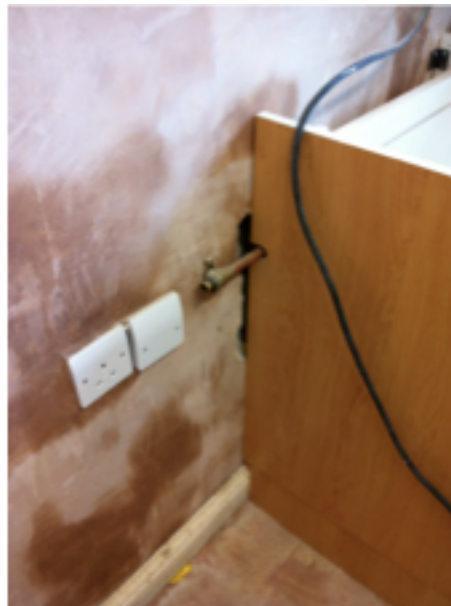
Figure 20 – Gas pipe relocated due to inaccurate drawing
