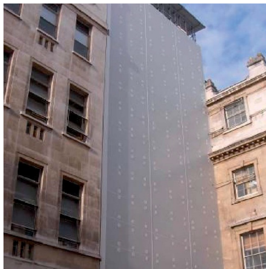
Figure 6 - Deconstructive 7 acoustic screen used to shield the children's intensive care unit at The Royal London Hospital (CE, 2007)
