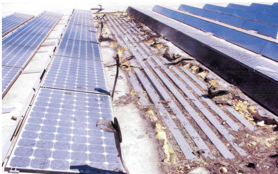
Figure 1.2 Fire hazard in a 383 kW PV array, in Bakersfield, California 2009 (Brooks, 2011)
