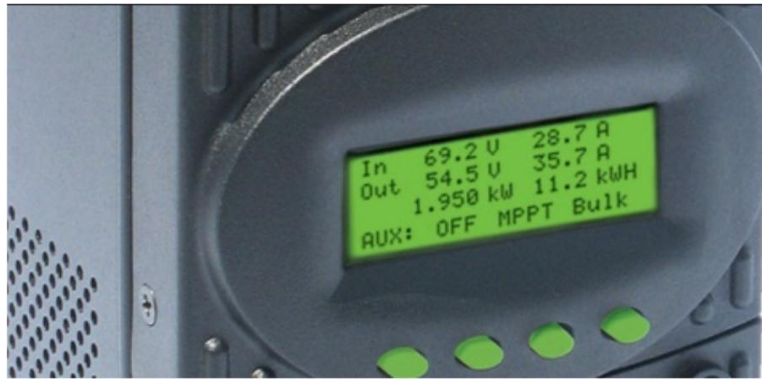
Figure 3.4 Image of the monitoring screen for FLEXmax 80 MPPT device
