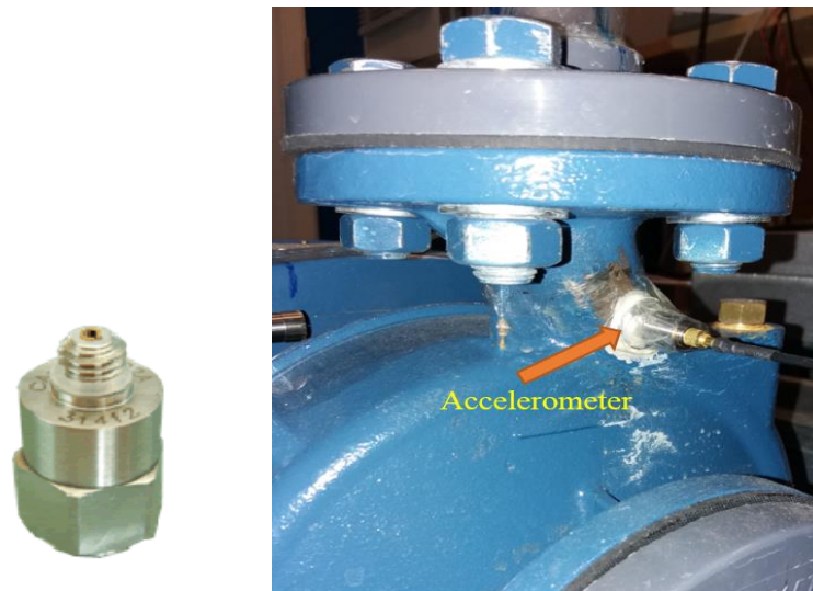
Figure 4-5: Accelerometer and its location on the centrifugal pump
